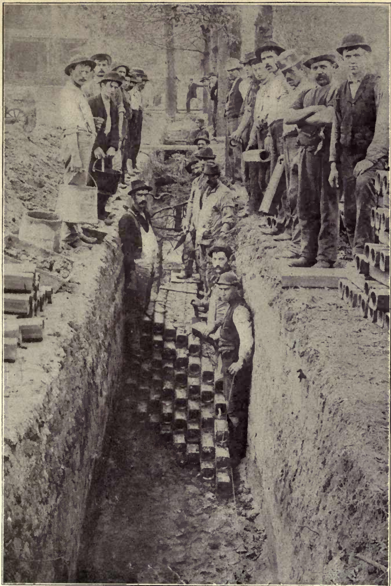
A SUBWAY LAID WITHOUT BOTTOM CONCRETE
